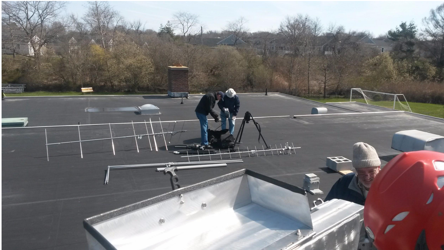
Gear being offloaded, and antenna assembly underway Jeff Greer (left), Jim Sammons (middle), and Paul Silverzweig (right)
