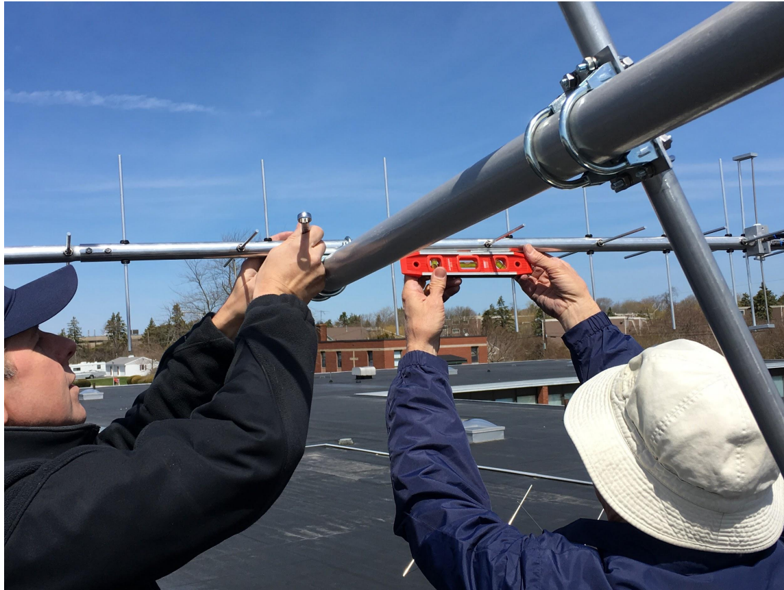
Installing Antennas & Making sure things are plumb (Jeff on left, Jim on right)
